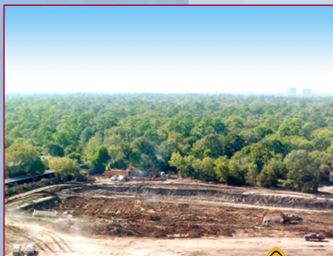
▲ Construction crews excavating the detention pond located at the southwest corner of the IH 10/Beltway 8 Interchange.
