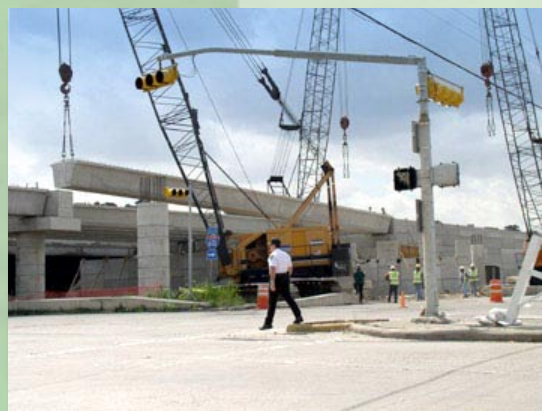
Placing of a beam for IH 610 southbound mainlane bridge. (at Memorial Dr. intersection)
