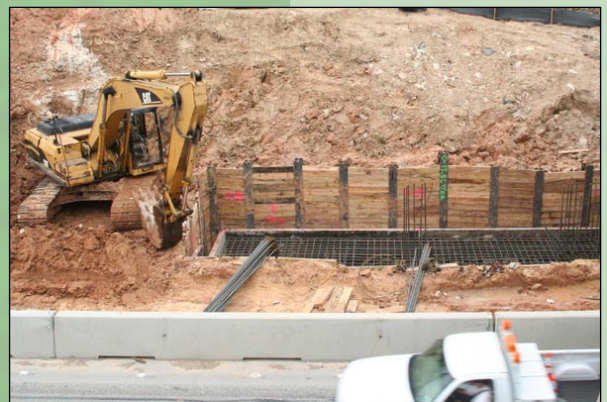
Contract G - Construction has begun on the temporary Union Pacific bridge on the north side of IH 10
