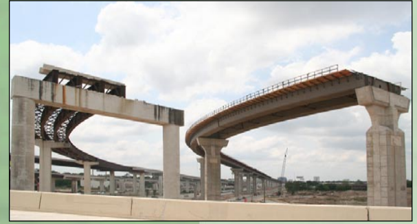
Contract D - The new Beltway 8 southbound to IH 10 westbound direct connector (DC H) is being constructed north of the old direct connector (looking west)
