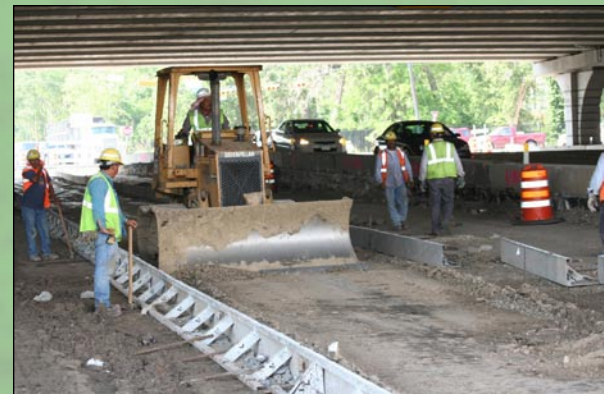
Contract C2 - Construction crews are working on the IH 10 eastbound to westbound U-turn at Dairy Ashford
