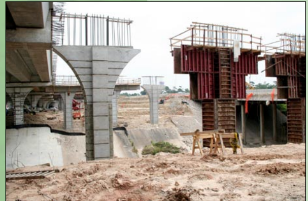
Contracts E1 and E2 - The contractor has completed several new columns for the new IH 10 mainlanes bridge over Wirt/Chimney Rock
