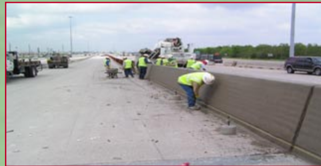
Contract B - Workers are finishing the surface of IH 10 center barrier near Barker Cypress.
