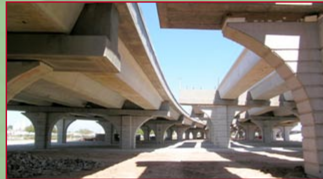
Contract A - View, looking east, of beams for the IH 10 eastbound mainlanes bridge over US 90 which were recently placed.
