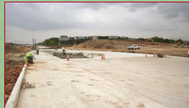
Contract C1 - Workers are completing the surface of the new IH 10 westbound frontage road east of Eldridge.
