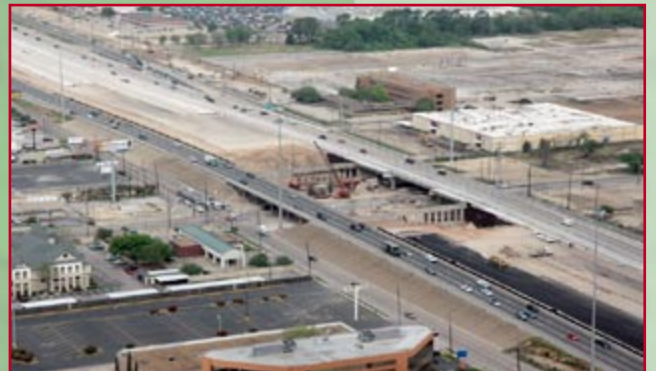
Contract E1 & E2 - Aerial view, looking east, of construction near the IH 10/Bunker Hill intersection.
