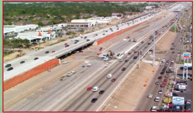
Contract C2 - Aerial view, looking east, of the new IH 10 westbound mainlanes north of the old westbound frontage road near Kirkwood.
