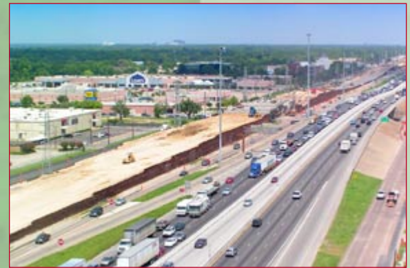
Contract E1 and E2—An aerial photo of construction along IH-10 near Bunker Hill (looking east)
