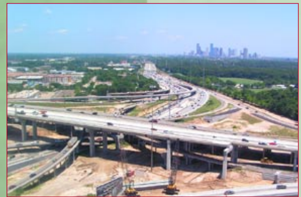
Contract F—Traffic was recently switched onto new IH-610 southbound mainlanes over IH-10
