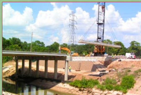
Contract C1—Placing a beam for new IH-10 westbound frontage road over Langham Creek
